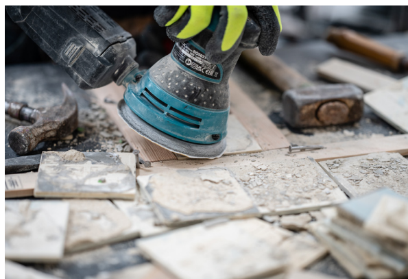
Dismantled tiles are cleaned then packaged for reuse at a later stage.
