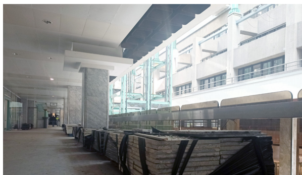
Large quantities of marble slabs were carefully dismantled and packaged by reuse operators. © Build-wise
