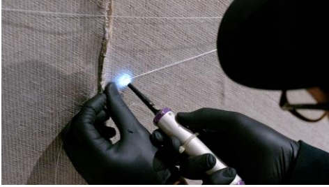
Structural Health Monitoring: artificial intelligence evaluates data from almost 100 sensors within the bridge in real time. The picture shows the installation of one of the fiber optic sensors.
