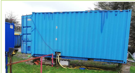
Figure 3: Struvia™ Pilot plant unit at Macroom WWTP (2)
