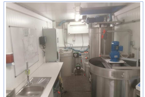
Figure 5: Internal View of Struvia™ Pilot plant (© Veolia)
