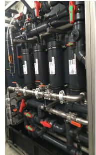
3 polypropylene hollow fibre membrane modules with 4 contactors each (212 m 2 per module) – 2 operated in series, 1 in stand-by ( 3M )
