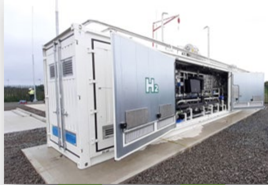
First green powered electrolyser on the island of Ireland
